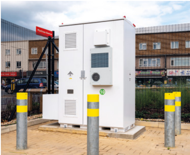
A battery storing rooftop solar energy at our Slough store.
