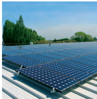
Solar panels, Twickenham
