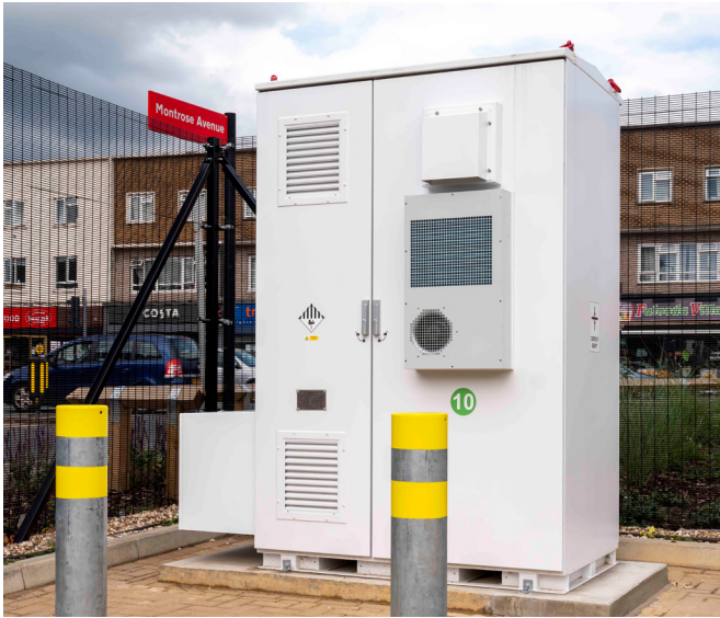
Battery storing rooftop solar energy at our Slough store
