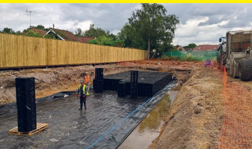
Attenuation tank for the SuDS infrastructure at our new store in Uxbridge being installed
