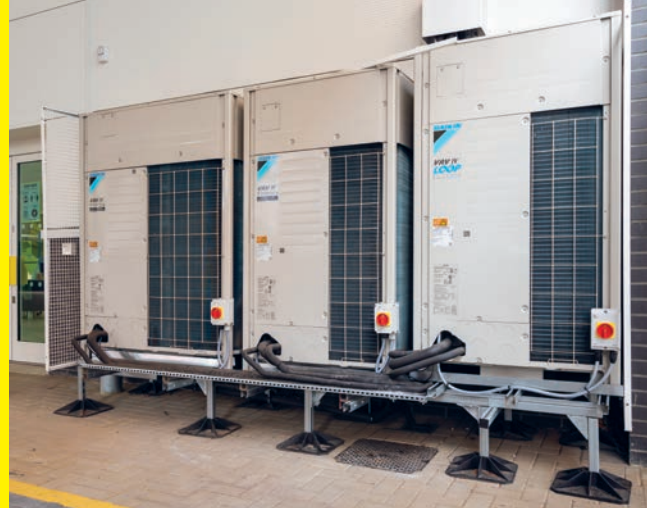
Air source heat pumps at our Battersea store.
